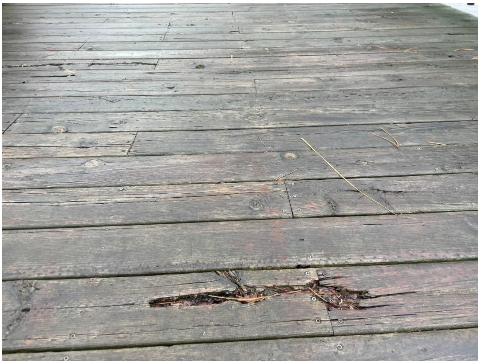
Figure 7 - Example of typical decking defects
