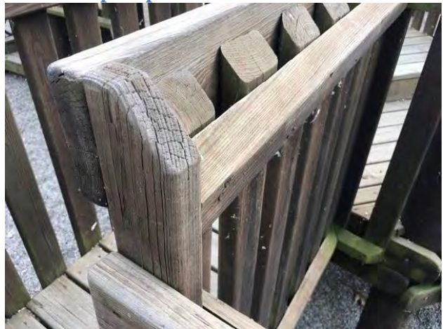
Handrail post picture #2
