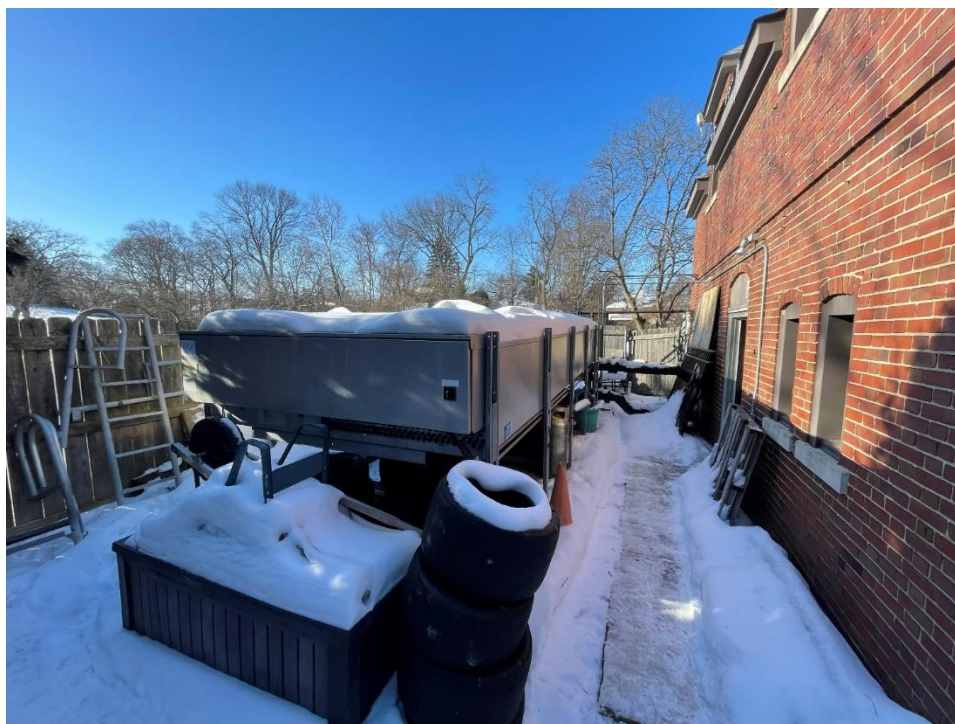
Figure 6 – External Condenser Unit
