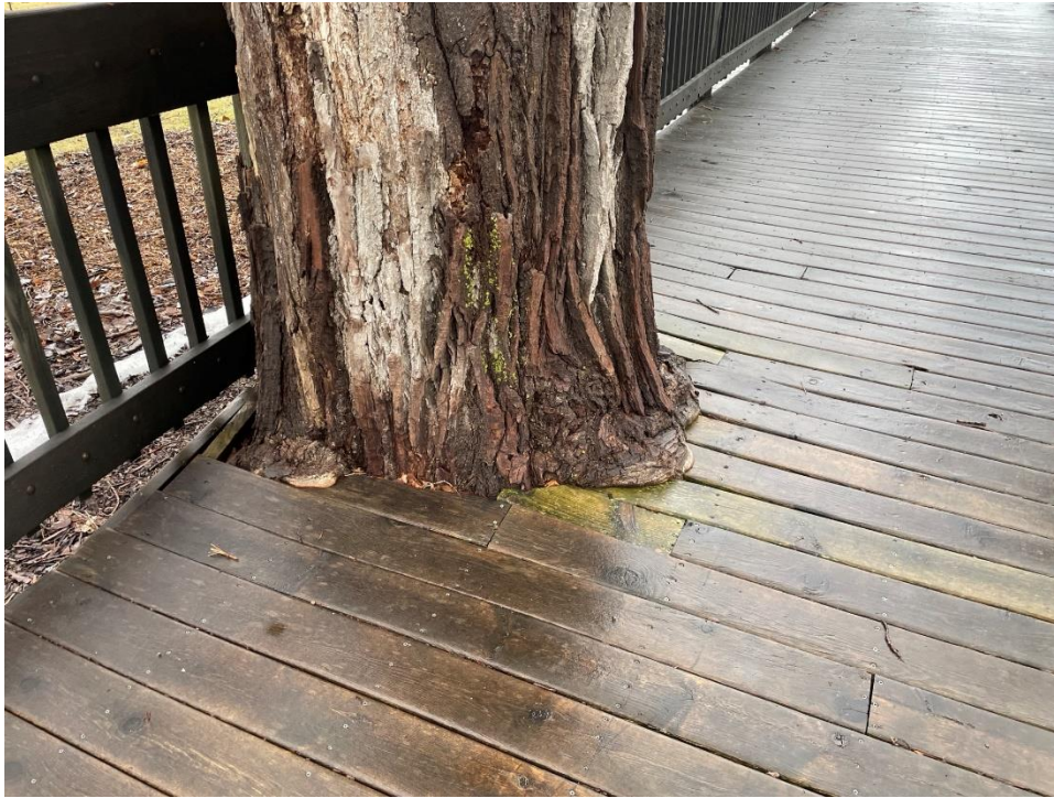
Figure 6 - Heaved Boardwalk at existing tree
