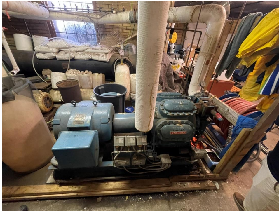
Figure 7 - Condenser No. 2 to be replaced
