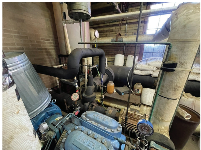
Brine Circulation System within Carriage House.
