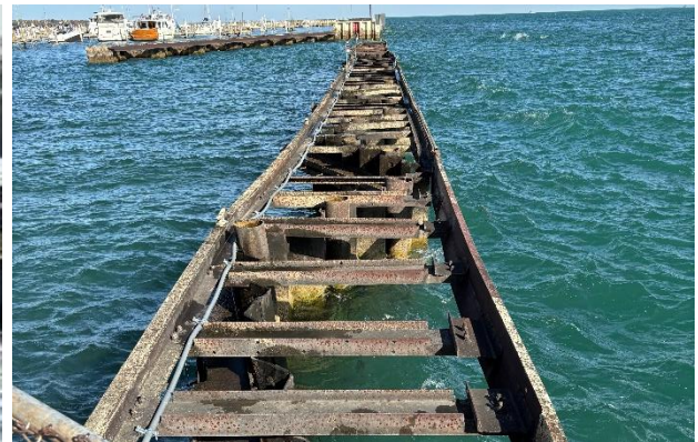
Figure 27: West entry wall from shore.
