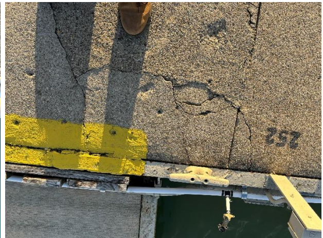
Figure 5: Cracking deck on Pier 2.
