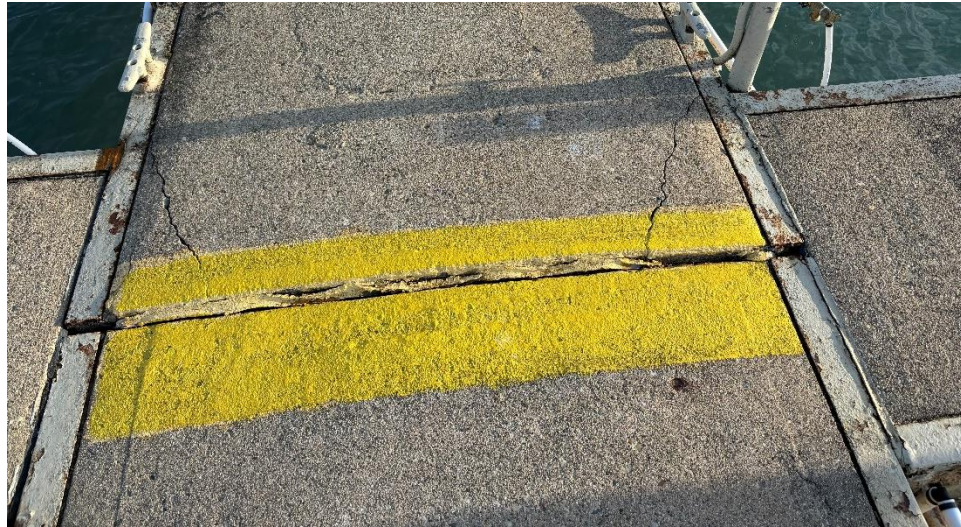
Figure 6: Bulging deck joint on Pier 4.
