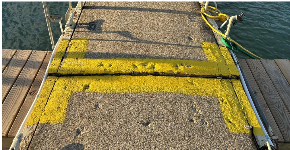
Figure 7: Bulging deck joint on Pier 2.
