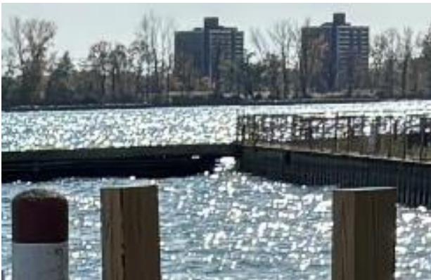
Figure 26: Missing section of west entry wall.
