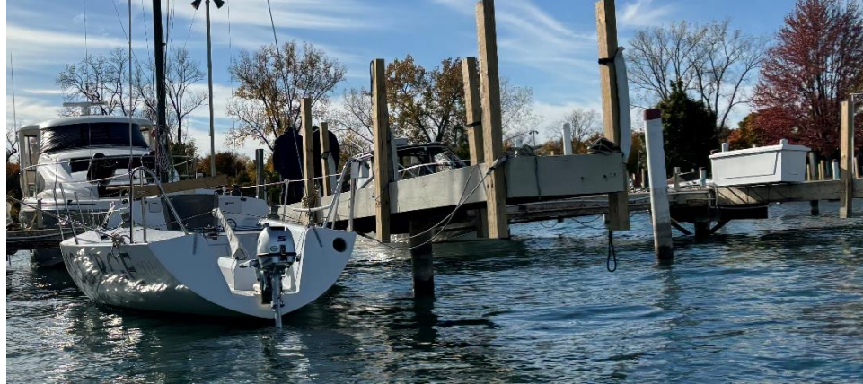
Figure 22: Heaved finger pier (Pier 4).
