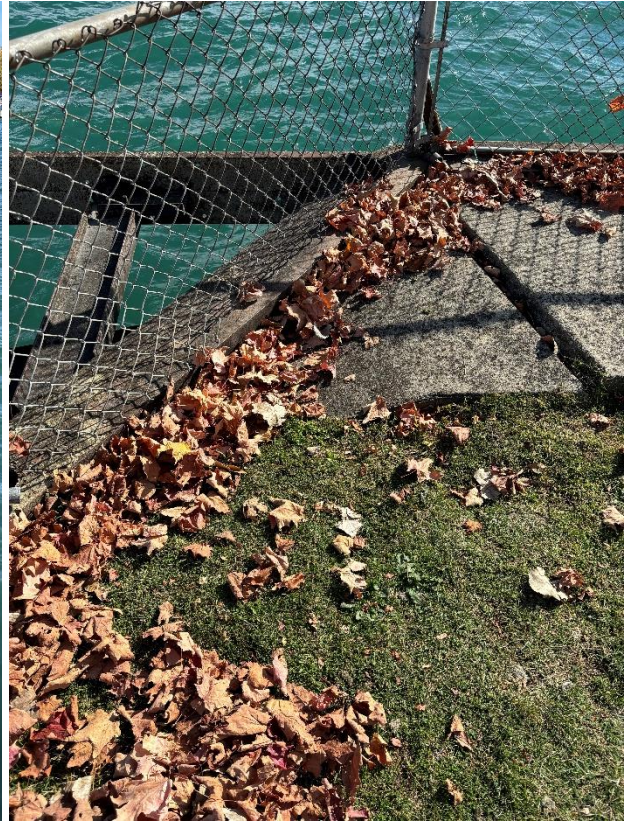
Figure 25: Settlement, south end of west seawall.
