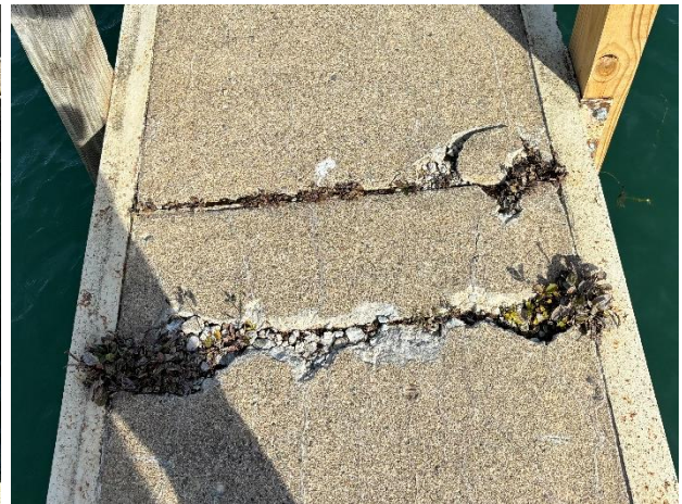
Figure 3: Spalling deck on Pier 4.
