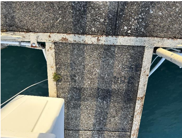
Figure 4: Weathered deck on Pier 3.
