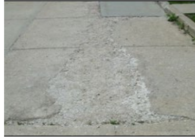
SPALLING GREATER THAN 75% OF FLAG
