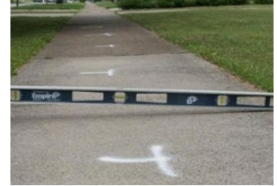
CROSS SLOPES GREATER THAN 2%
