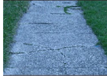
CRACKS 3/8" MAX WIDTH
