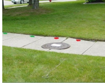
DEFECT DUE TO MANHOLE COVER
