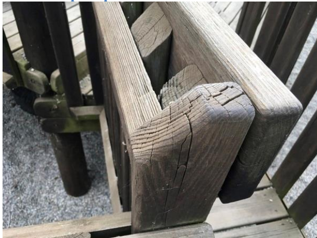
Handrail post picture #1
