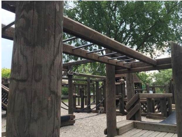
Horizontal Ladder picture #1
