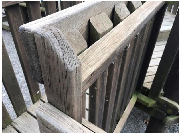
Handrail post picture #2
